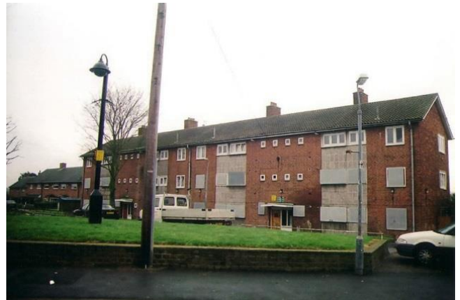
Figure. Steel security window grilles; CCTV camera. Birmingham, UK (photo: Phil Jones)
